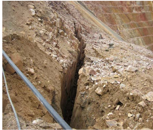
Figura 6. Tensile crack in a slope of the Tinyag mine
