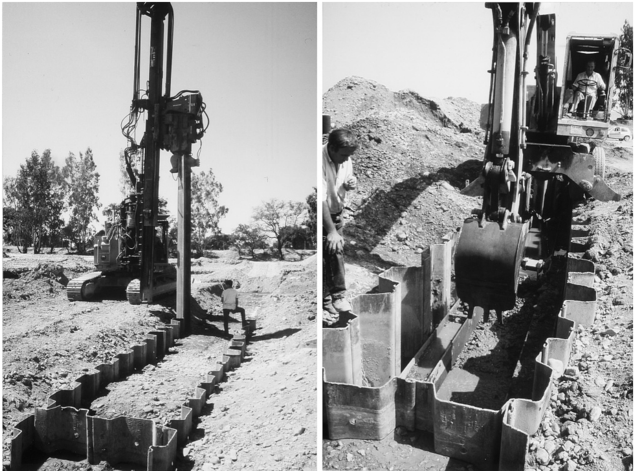
Fig. 3. Permeable Reactive Barrier construction. Left: installing steel sheet piles to hold the alluvial walls. Right: backhoe excavation prior to filling with the reactive material.
