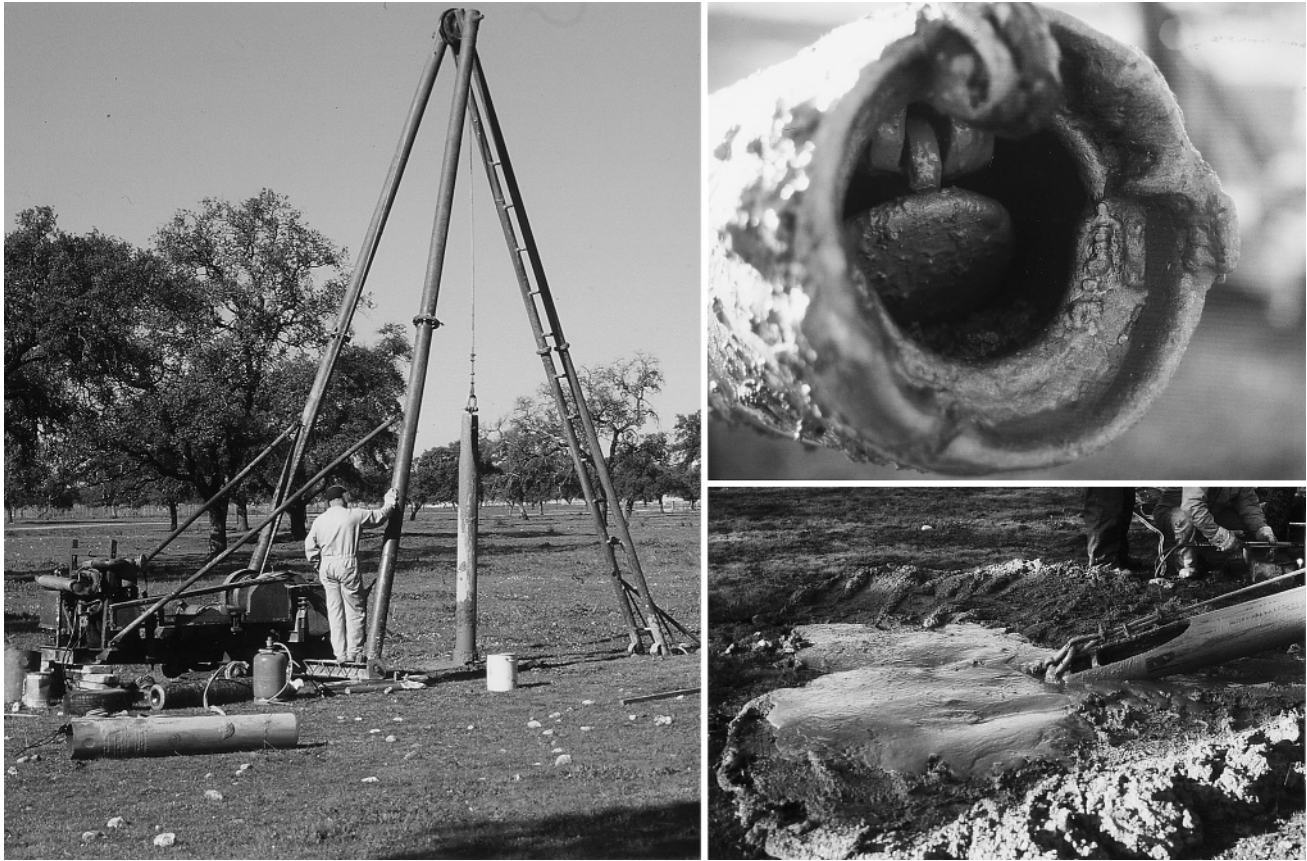
Fig. 4. Drilling method used to study the alluvial deposits of the Agrio River: Left: Tripod and hanging steel bailer. Right-above: detail of the valve in the lower end of the bailer that facilitates retention of cuttings within the cylinder. Right-below: bailer emptying. Deposited material is a mixture of water and broken alluvium, sometimes with fragments of unaltered soil.
